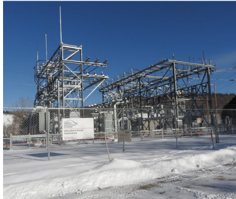
Green Mountain Power's Woodford Road Substation in Vermont | © RTO Insider
