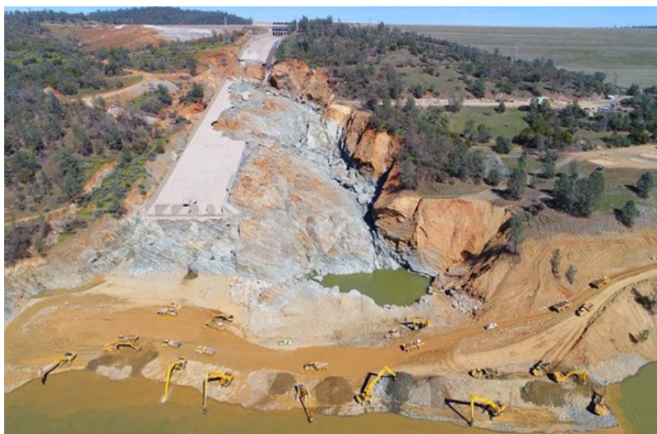
Ultimate damage at the service spillway | Independent Forensic Team Report
